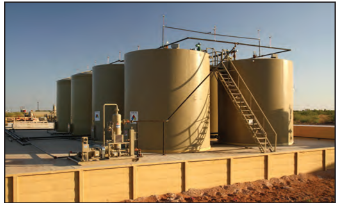
Secondary containment structure-
